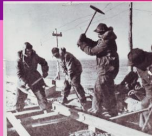
FIRST RAIL of a short line for unloading equipment at Seven Islands is tackled down to 500 men each task of distributing $8,000,000 worth of equipment along the first 40 miles of the line for spring track-laying. Editorial Director Special, South American & Co. Ltd.
